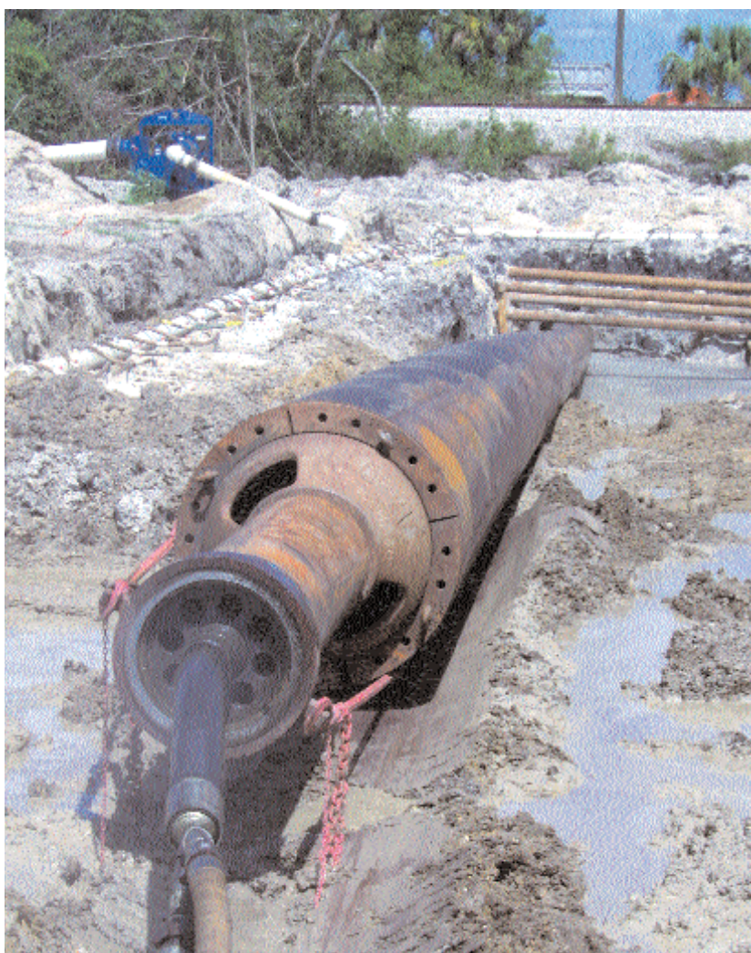
An American Augers DD-140 was used in conjunction with a TT Technologies 18-in. Grundoram Goliath pipe ramming tool attached to the end of each pipe.
